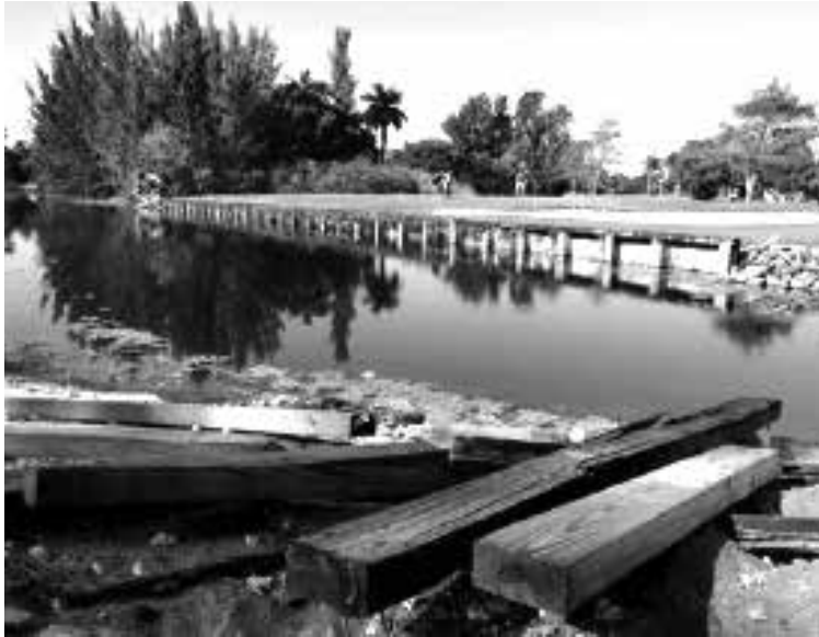
Rotten and damaged boards are shown at Orangebrook Golf Course on Tuesday. (Amy Beth Bennett/South Florida Sun Sentinel)
